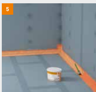
5 Immediately apply a coating of fermacell Waterproofing Application to the Sealing Tape
